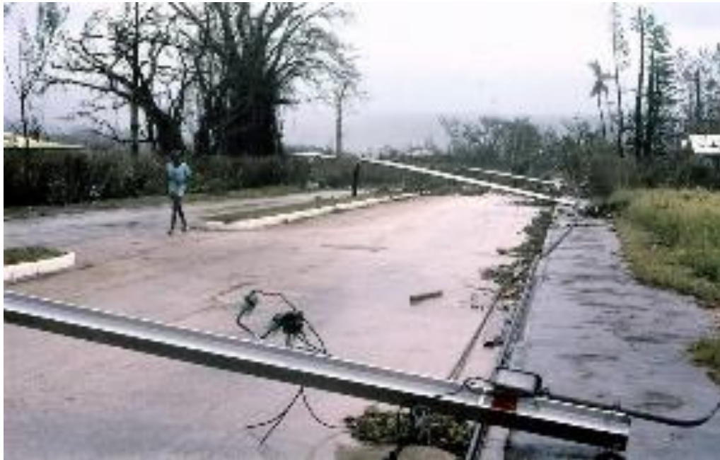
Figure 1.5 Cyclone Uma, February 1987: in Port Vila, violent winds have bent these reinforced steel utility poles down to the ground
